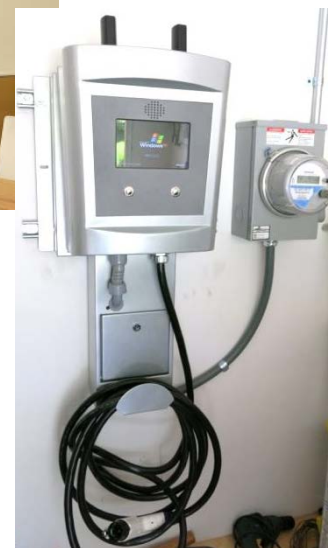
Electric Vehicle Charging Station
