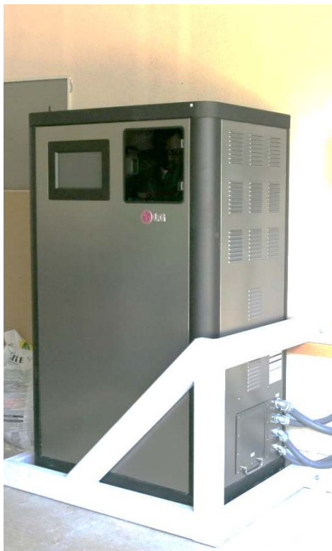
Residential Energy Storage Unit (Battery)
